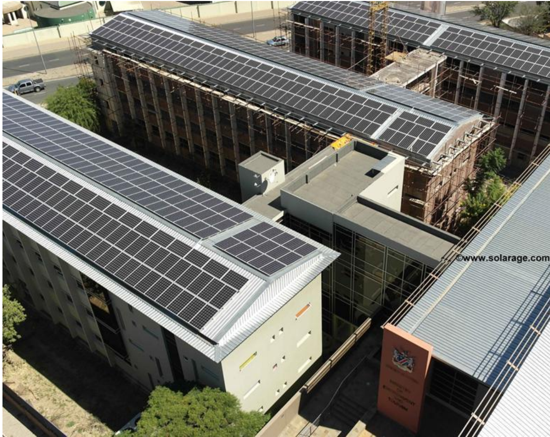
MET Head office and its new roof mounted photovoltaic system
